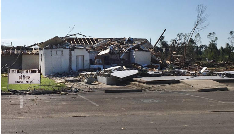
First Baptist Church of Moss, Miss., was destroyed when tornadoes swept through several Southern states Easter Sunday and early Monday. Photo submitted by pastor Tony Johnson
